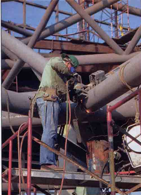
Connections involved three and four pipes.
