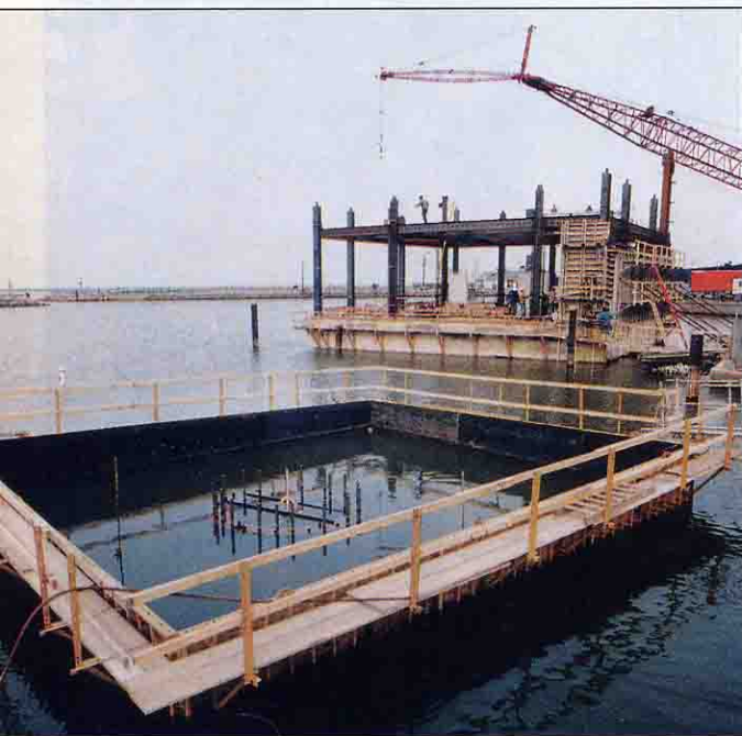
Forms for pile caps create a cofferdam to place concrete in lake.
