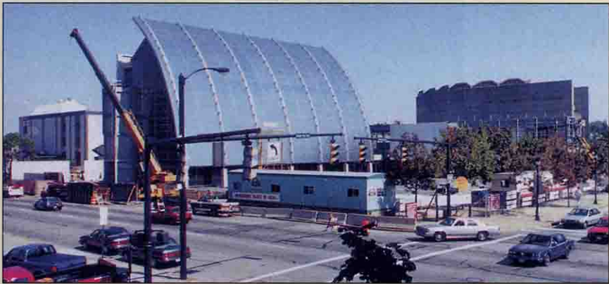
Stainless steel sail at new home of Inventors Hall of Fame in Akron creates an uplifting spirit.
