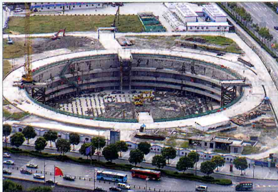
▲ Big Mat. Concrete mat for tower on course for completion next month.
