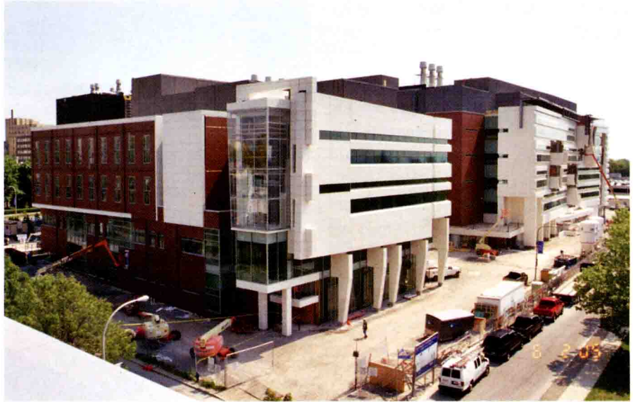
To meet a fast schedule, the project team pursued early bid packages in 2003 for excavation, foundation concrete, underground plumbing, and structural steel. (Photo by Noreen Ersing/Cutting Edge Photo).
