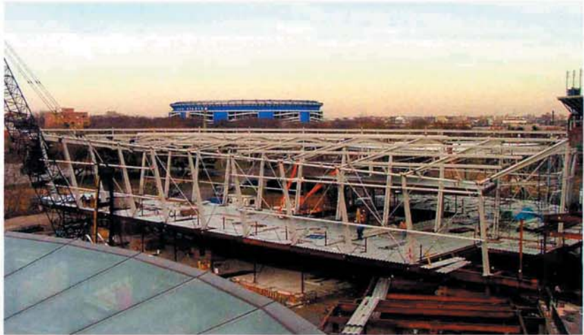
The Hall of Light consists of exposed structural steel rolled members, pipes, rods, tubes, and structural strand cable that are both design and structural elements of the building.
