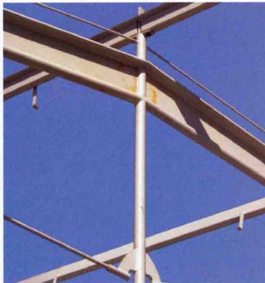
MIDDLE RIGHT The king post trusses are composed of cut wide flange beams, 4-inch pipes, and 1/4-inch-diameter high-strength rods.
