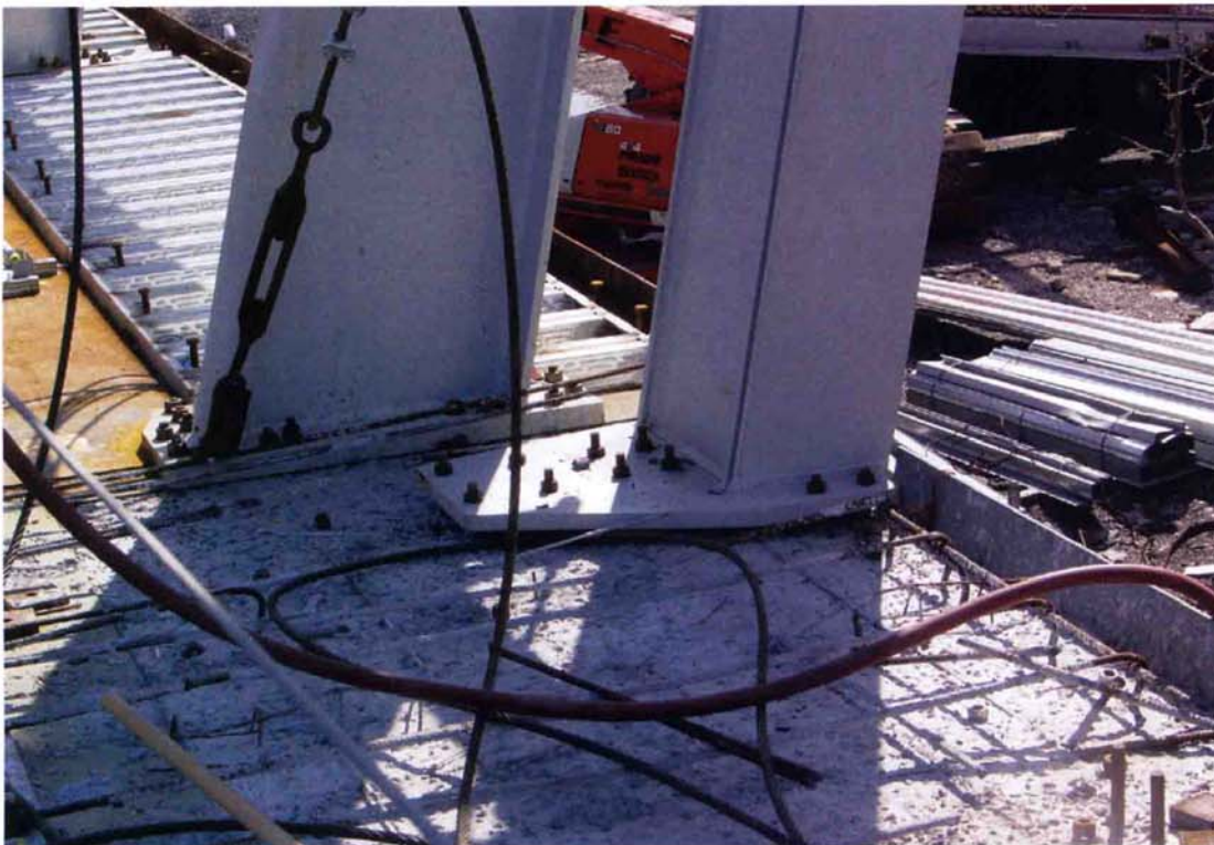
BOTTOM The structure's primary bracing against lateral forces takes place at moment connections between floor girders and column bases.
