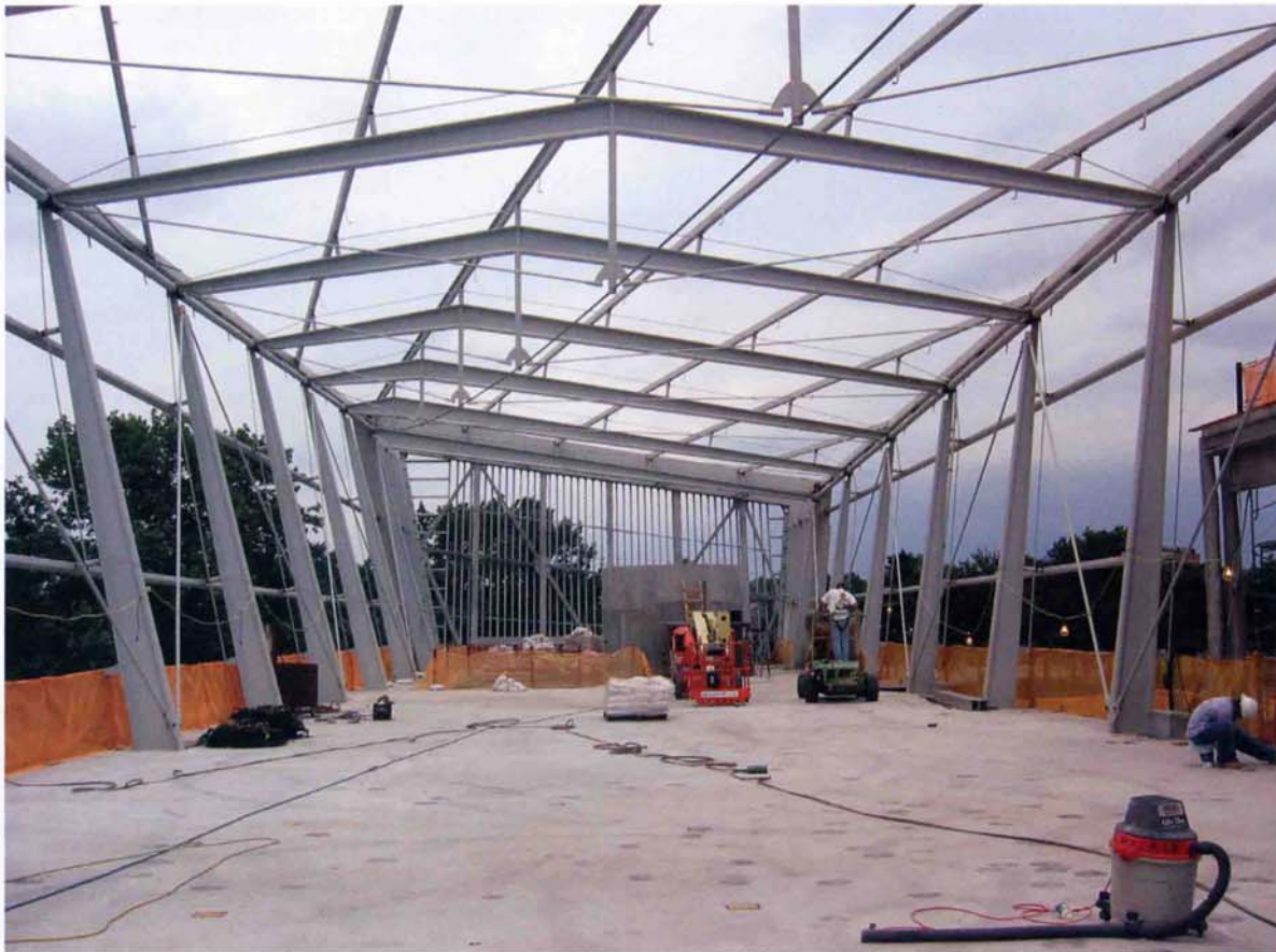
PREVIOUS The addition's expressive steel structure and translucent cladding give the Hall its name.
