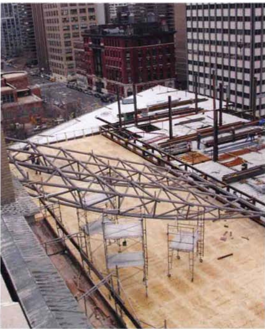
ABOVE The skylight's bow trusses bolt to the addition. Hangars tying back to the existing steel frame connect it to the historic building, while allowing for independent lateral movement in case of seismic activity.
